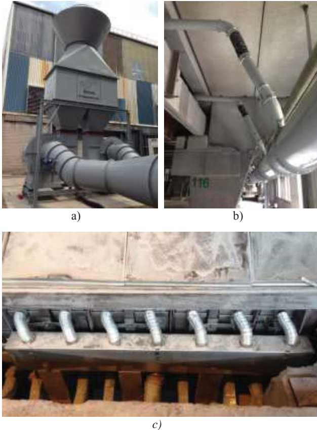
Figure 3- SHE trial installation details showing a) Redundant dual-fan system and exhaust stack with silencer, b) branch ducts to pot side in basement, c) SHE units connected to distribution manifold box on pot sidewall
